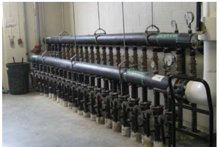
A ground source heat pump reduces energy costs
