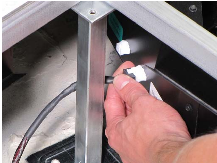
Figure 17 - Connection of temperature sensor tree
