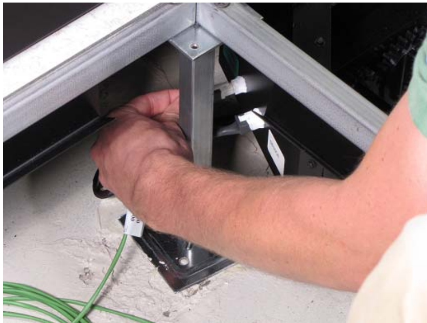
Figure 13 - Powering SmartAire from neighboring unit
