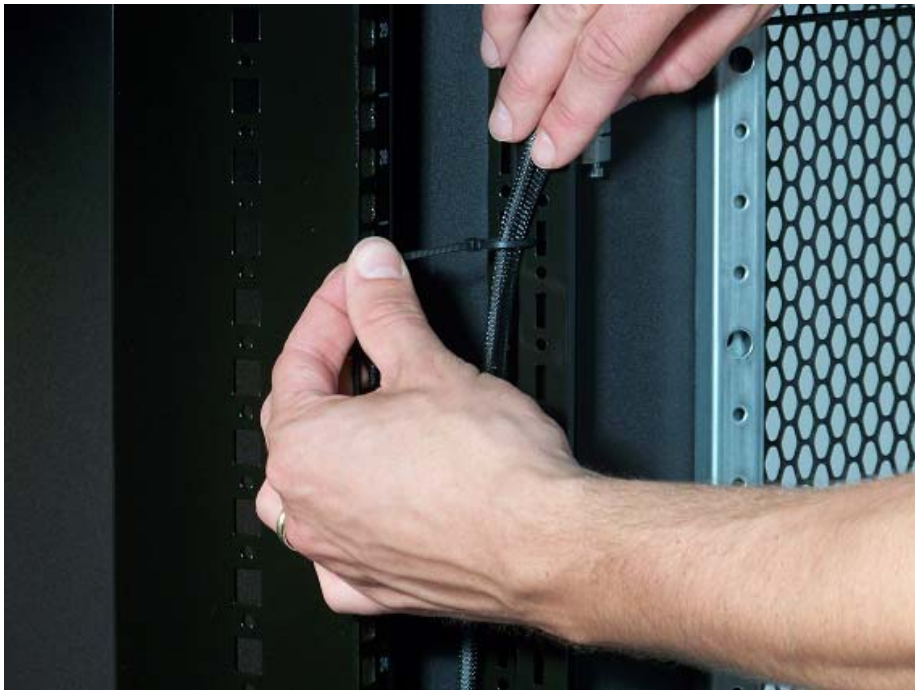
Figure 20 - Securing Sensor Tree to Rack with Sufficient Slack for Door Operation
