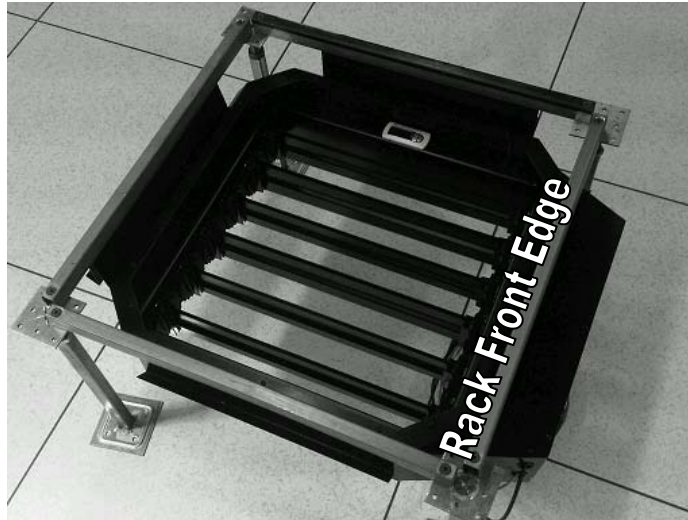
Figure 16 - SmartAire™ Unit Installed on hangers
