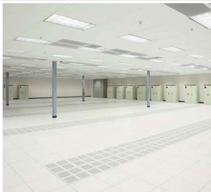
The 30 inch raised floor at 1500 Space Park houses the underfloor HVAC, cables and sprinkler system.
